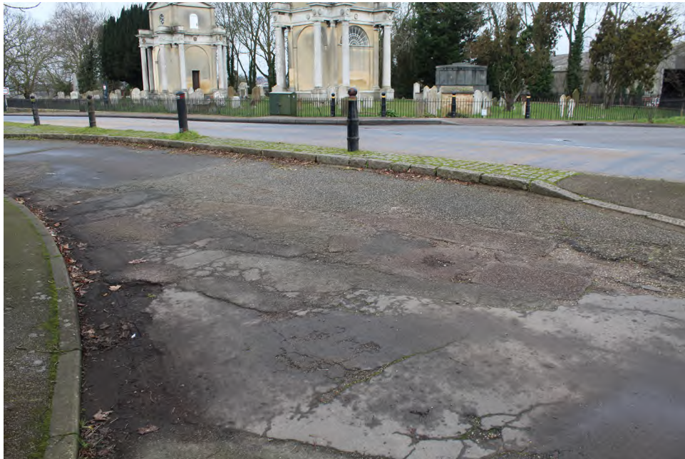
Figure 162 Poor surface treatments opposite Mistley Towers
