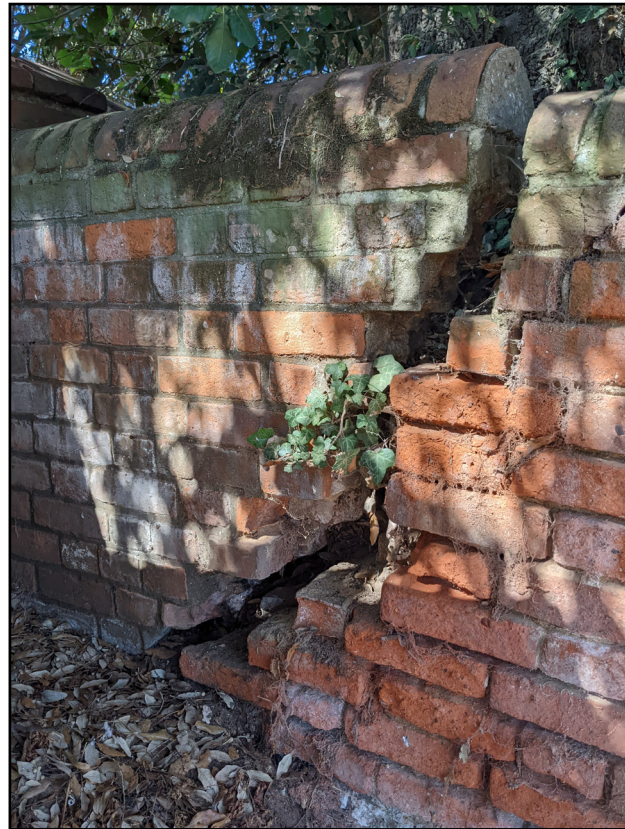
Figure 24 Damage to Brightlingsea Hall boundary wall
